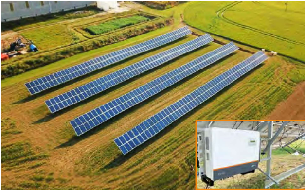
Lincolnshire, UK 140kW
