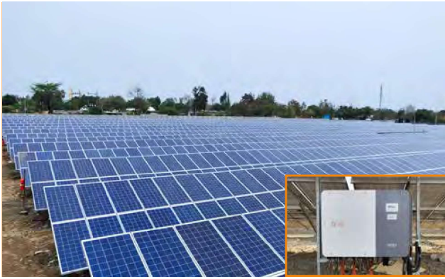
Latur Maharashtra, India 2.8MW
