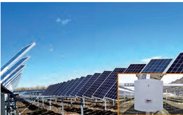
Hebei Zhangbei Agricultural-photovoltaic hybrid PV plant 50MW
