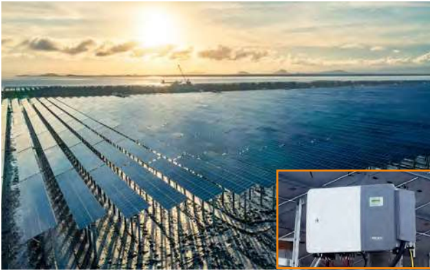
Zhejiang Ningbo Tidal Flat PV Power Project 300MW
