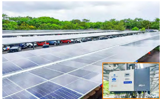
Carport project, India 6.2MW
