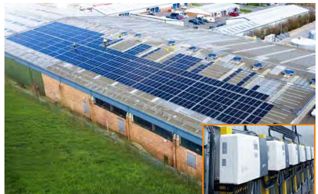
Faerch Plast Project, UK 2MW
