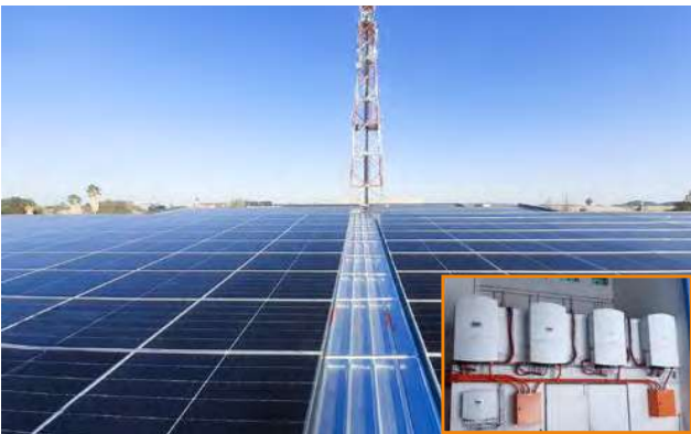
SolWorx Project, Namibia 272kW
