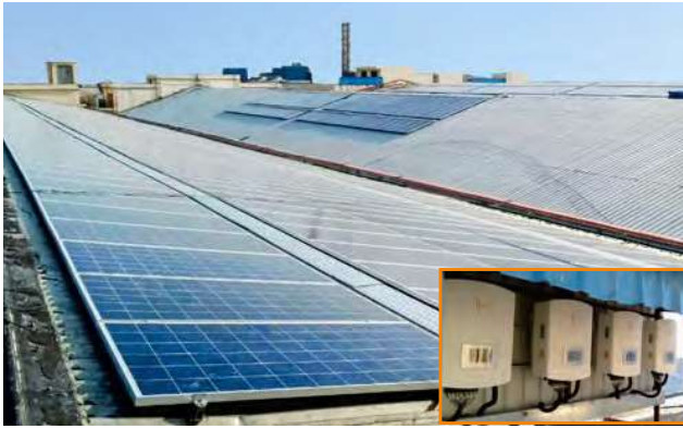
RSWM, India 3.6MW
