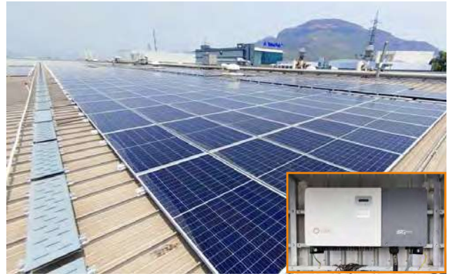
Tetra Pak Project, India 1MW
