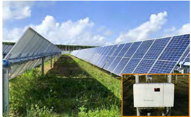
Vitoria Project, Brazil 2.5MW
